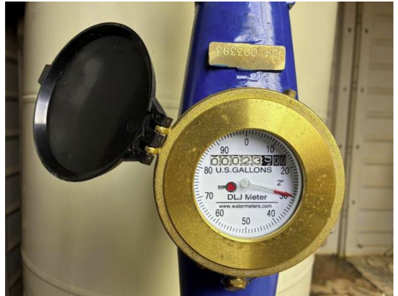
Figure 15. Water well meter
